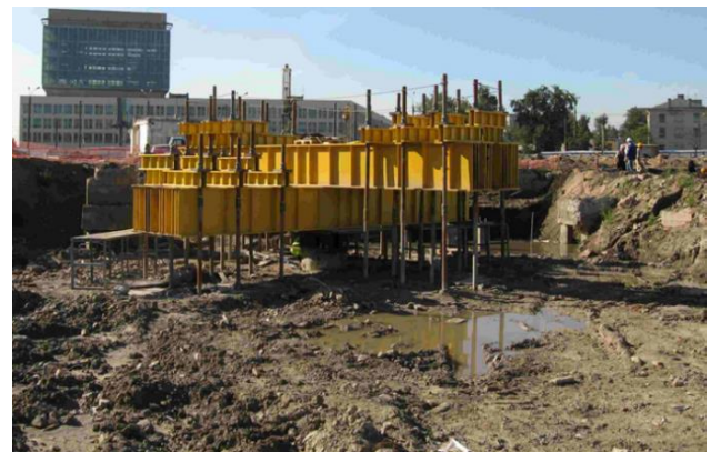
Figure 3. 30 MN top down reaction beams on a barrette test with multiple anchor piles (Fugro).
